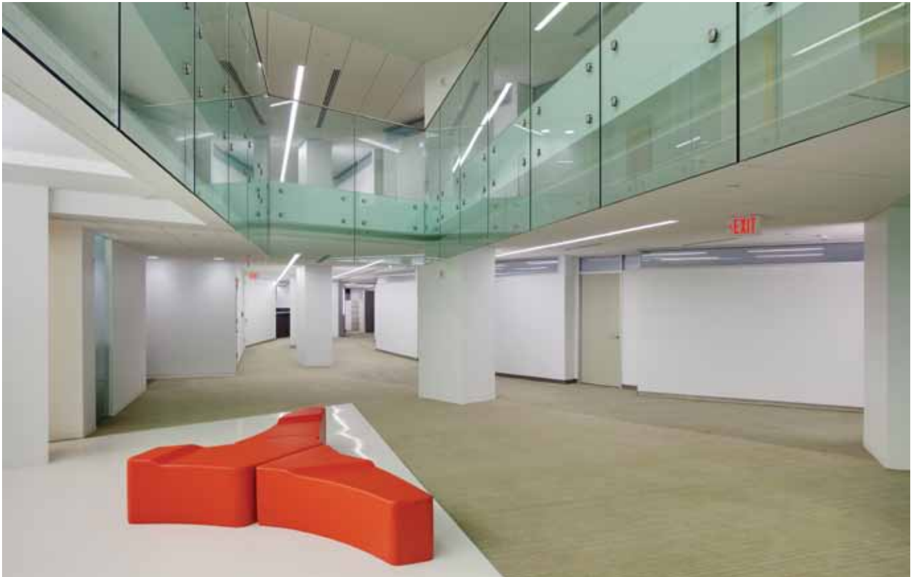
The ceiling between the fourth and fifth floors was removed to create “vertical connectivity” between the two floors.
